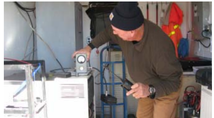
Randy W7RJB checking the power out of the Repeater.
