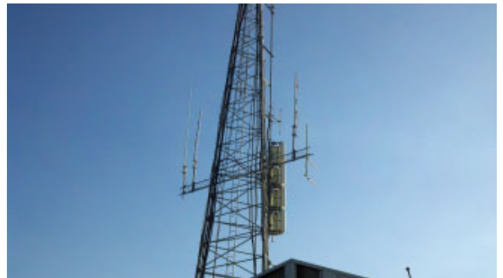
Usery Mountain Antennas
