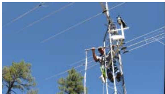
W7RJB Randy installing a way to pull up wire antennas from the ground.
