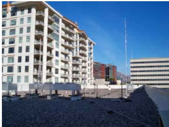
The antennas on the Red Cross Roof
